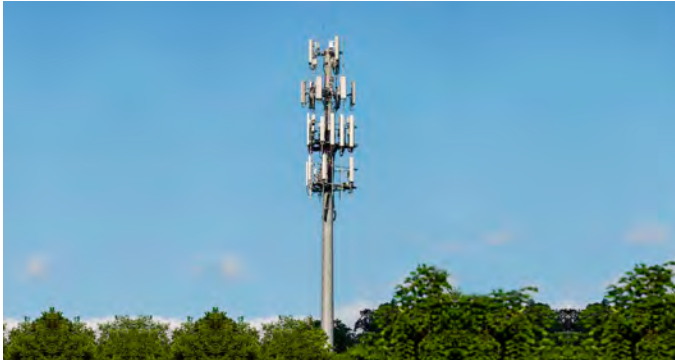
FIGURE 12. Cell Tower Using Co-Located Antenna Systems.
