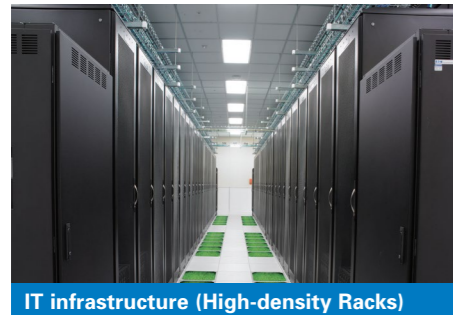
IT infrastructure (High-density Racks)
