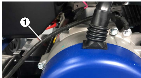
Figure 5 - Locating Negative (-) Cable
